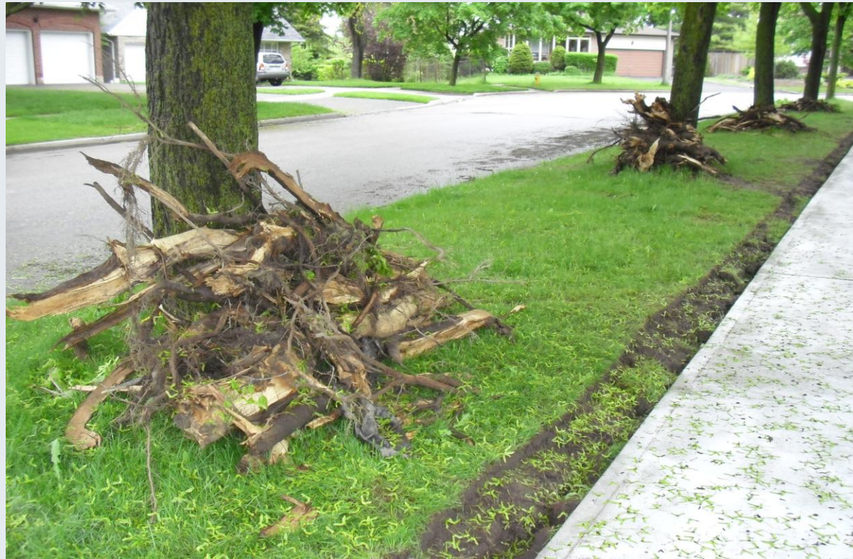
Sidewalk replacement due to damage from tree roots Scarborough 2011
